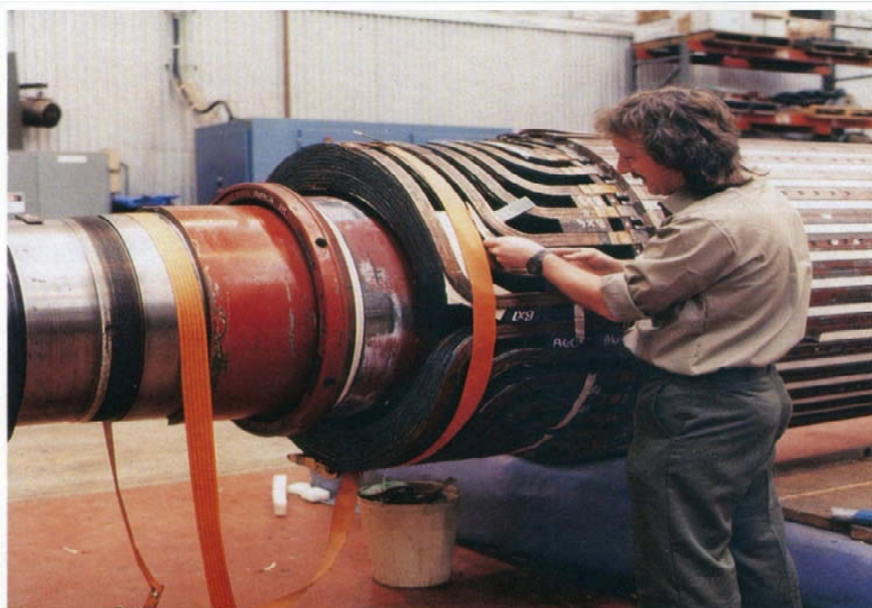
Repairs to the overhead insulation of this 200MW generator rotor were carried out by experienced tradesmen working on shift to ensure the earliest possible return to service.
