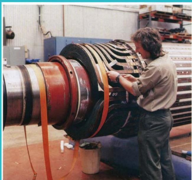
Repairs to the overhead insulation of this 200MW generator rotor were carried out by experienced tradesmen working on shift to ensure the earliest possible return to service.
